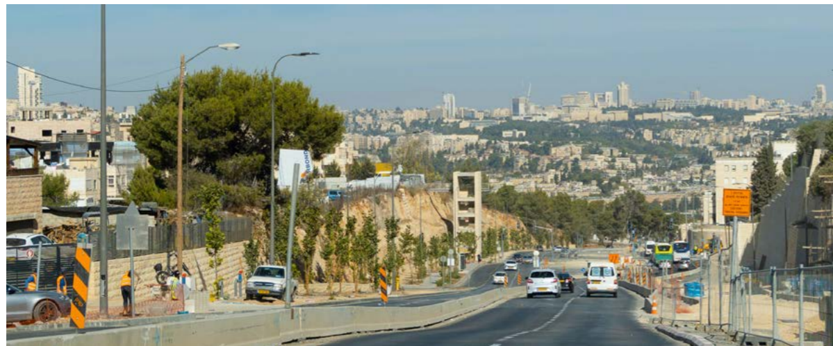
Fig. 258. Dov Yosef Street in the Sharafat neighborhood section. A vertical staircase still under construction will connect the neighborhood with the planned station
