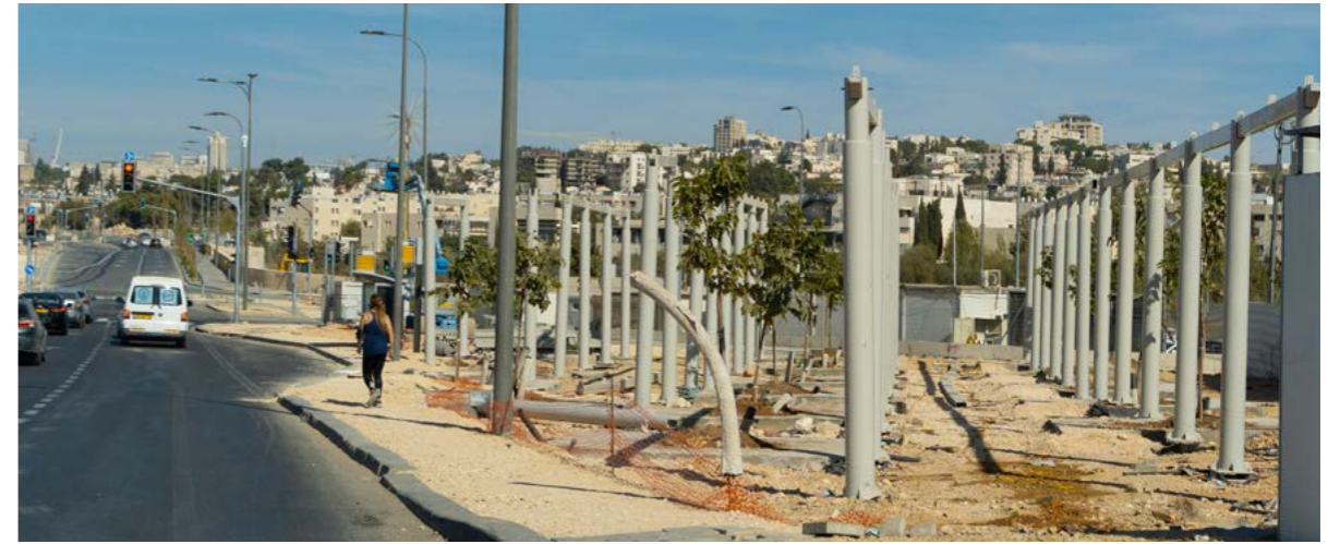
Fig. 260. The new meeting place and massive pergola adjacent to Beit Safafa's future station is under construction
