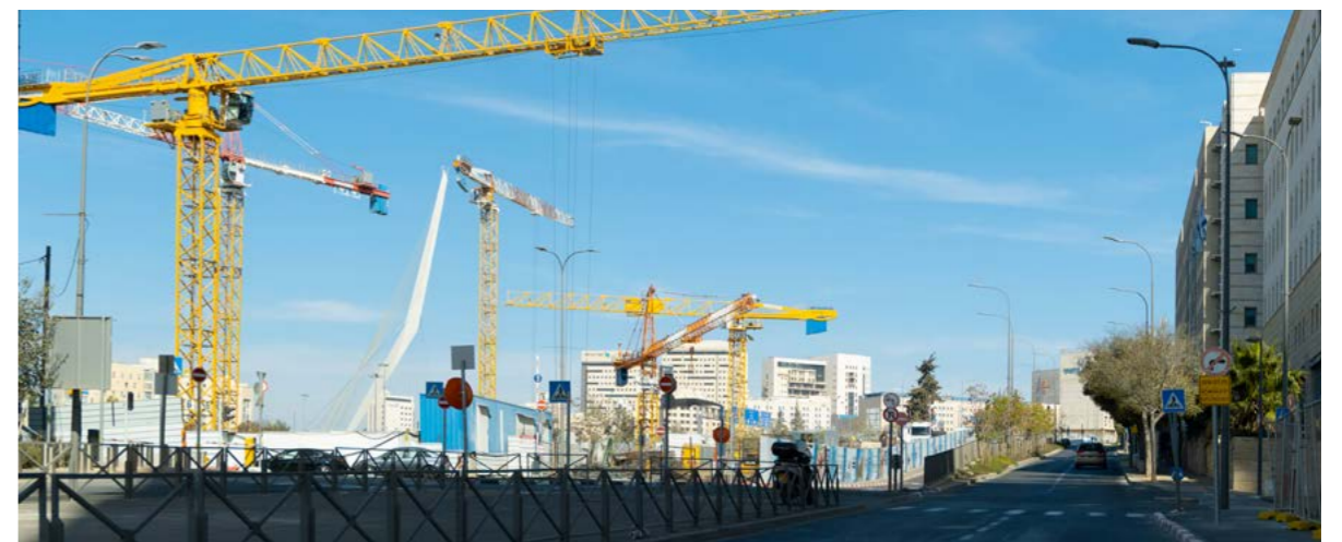
Fig. 267. Going up Natanel Lorch Street: the building cranes to the left mark the site of the future Green Line underground depot and government building complex, another mega-project of the practice
