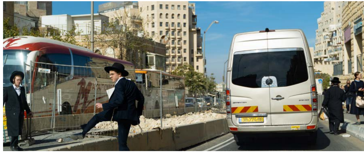
Fig. 268. The construction activities along Shamgar Street cause disruptions to the urban functioning of the street
