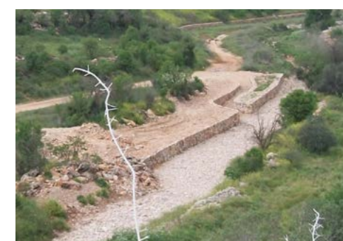
Fig. 22. In the Soreq stream bed rehabilitation, solid stones of different sizes were used for the thick walls lining the stream bed, to withstand enormous lateral water pressure during flood events, 2016
